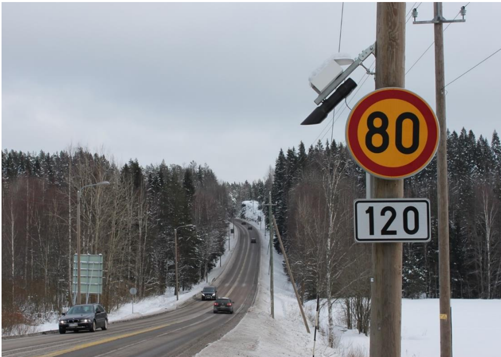
Figure 1. The compact road weather station installed on a wooden street light pole. The cabinet is on the other side of the pole at the height of the traffic signs.
