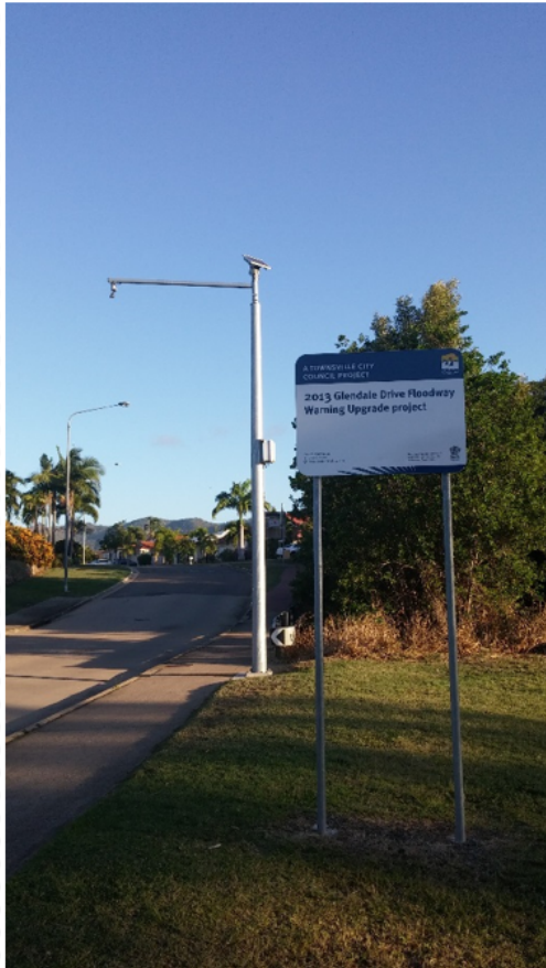
Figure 6: Radar Roadway Flood Monitoring System installed at the Glendale Drive floodway in Townsville.
